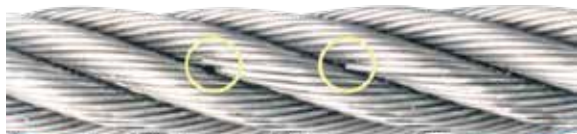
Figure 3: Example of valley wire breaks (source: ISO 4309)
